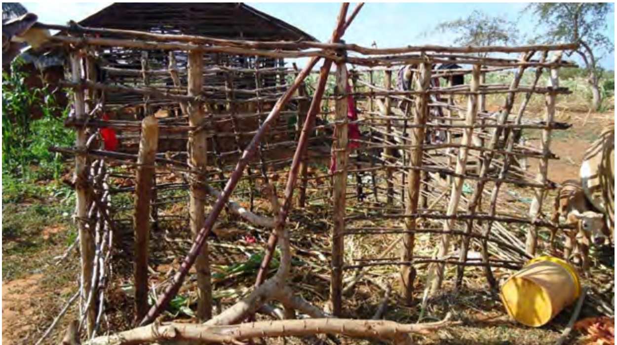
Reconstruction of destroyed Pokomo houses at Kilelengwani village. Photo: Patrick Bonyonte/KNCHR, February 2014
